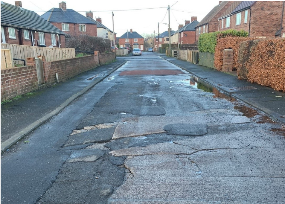
Image of poor road surface and road hump on Margaret Street
